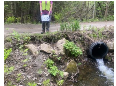
An unstable inlet/outlet around a culvert on a private gravel road
